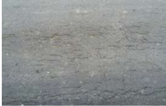
Gambar 3. Retak Halus / Hair Cracking
