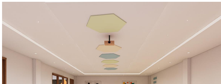
Gambar 4. 26. Penerapan Lampu Downlight
