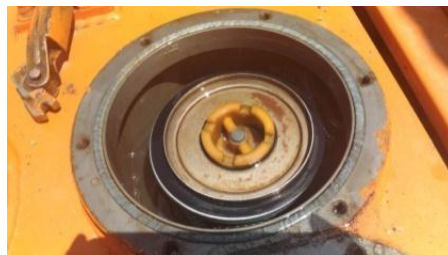
Gambar 13 Kondisi oil hydraulic .
